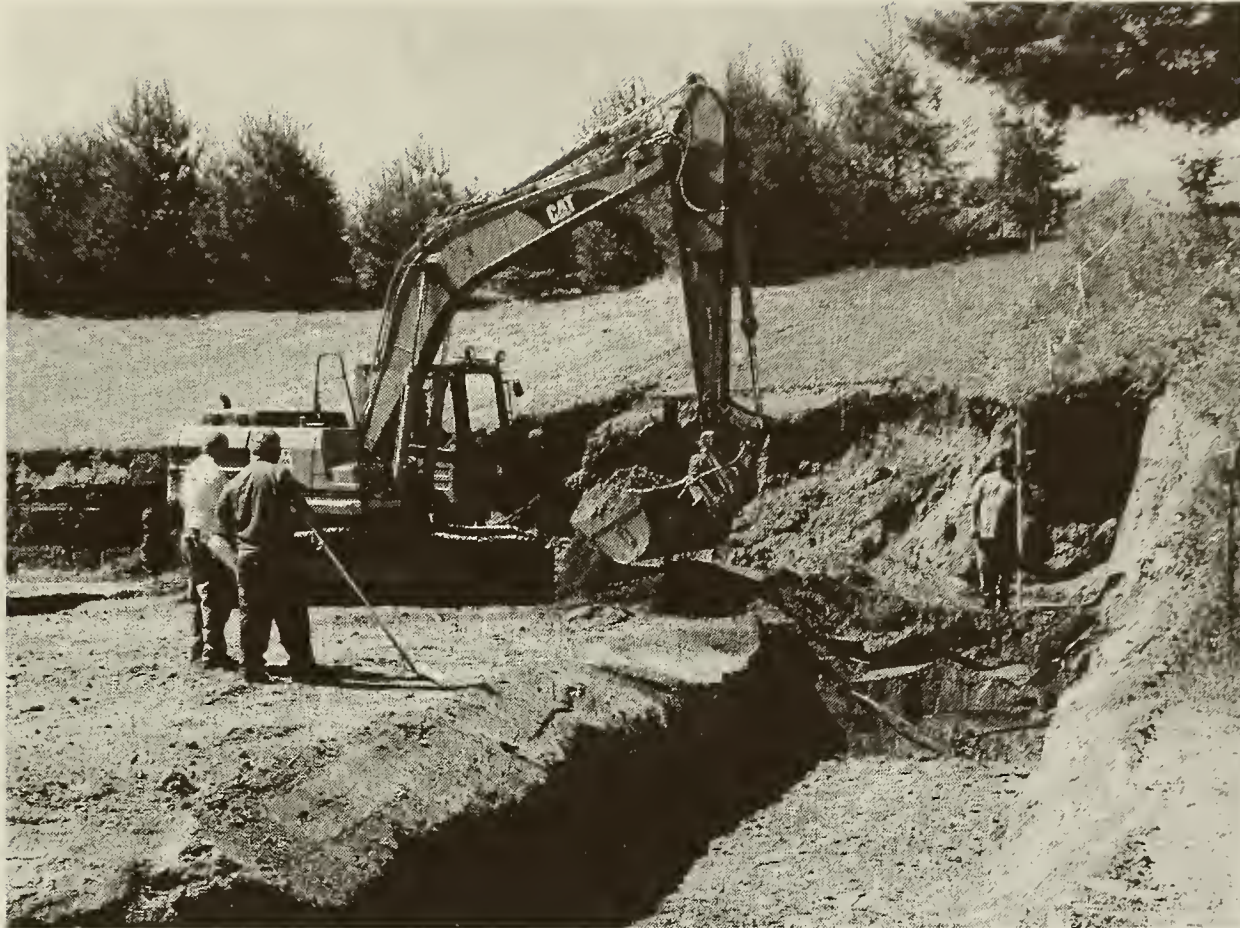
June 21, 2004, Excavation by Derby Mountain Construction of Lyme, NH (assisted by the Lyme Highway Department).
